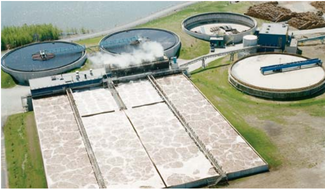
Secondary effluent treatment system - Trois-Rivières, Québec
